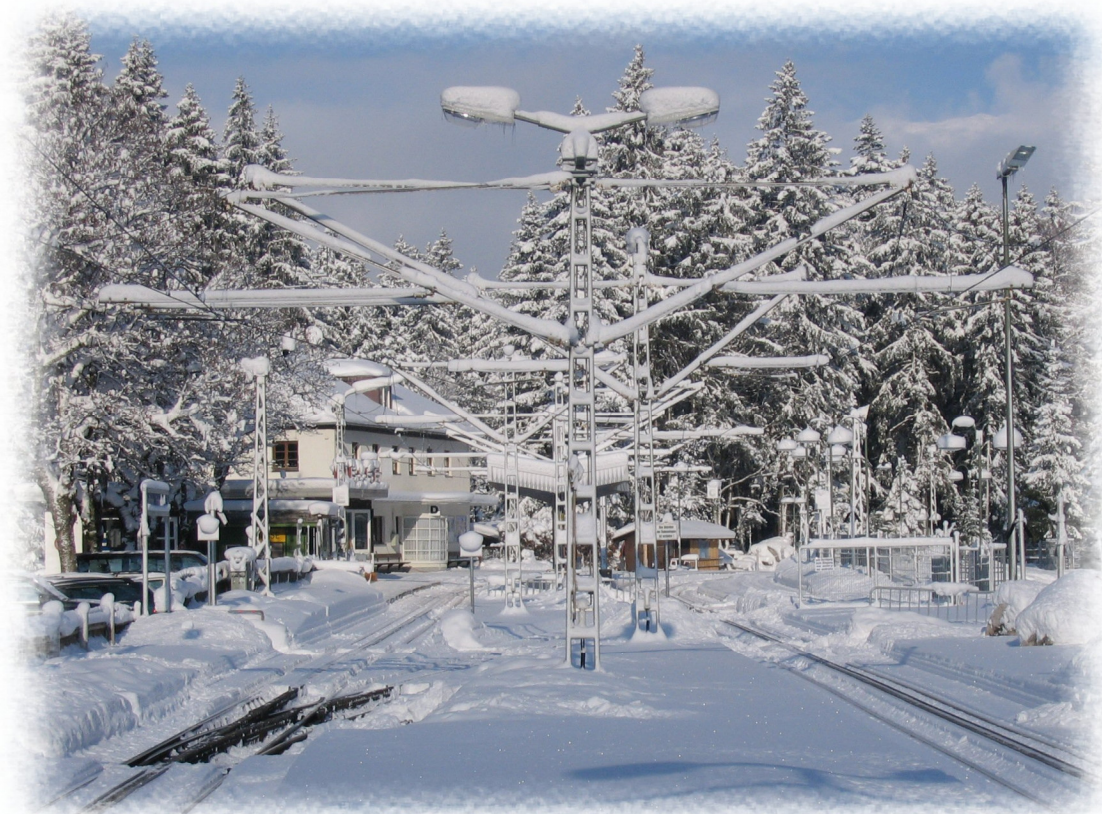
Wolff point heating system at Eibsee station submontane of germany ´s highest mountain the Zugspitze Picture with kind permission of Bayrische Zugspitzbahn
